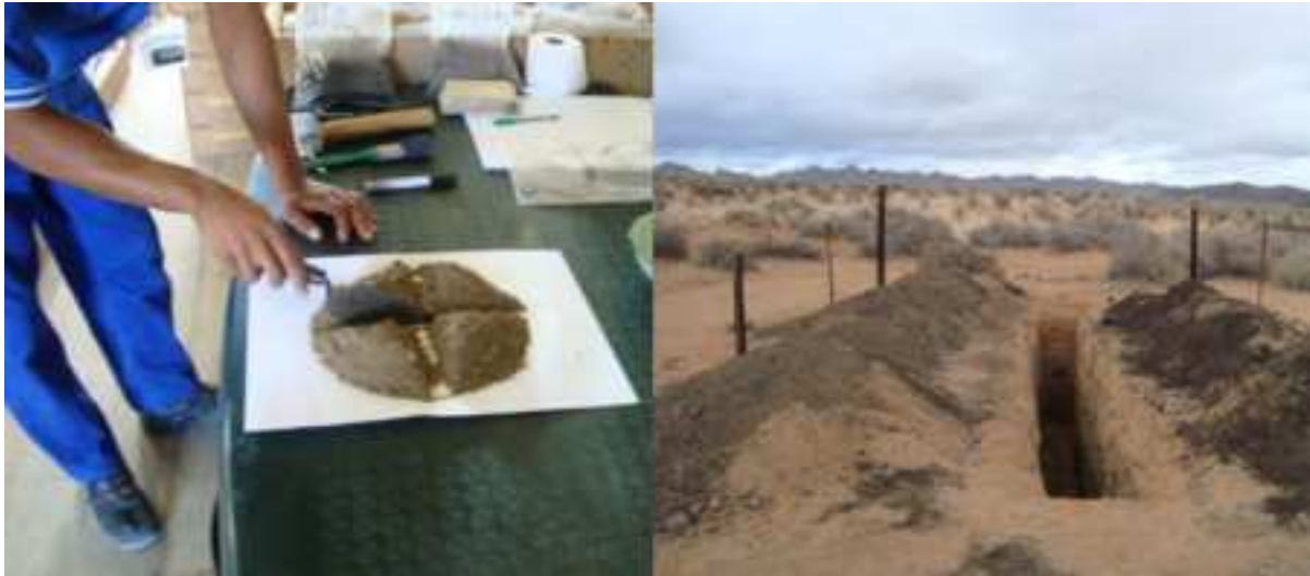
Figure 6-2. Right: Trench at Henkries Central. Left: cone and quartering of channel samples prior to pulverising and (portable) XRF analysis..
